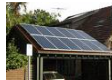
Solar Roof Top
